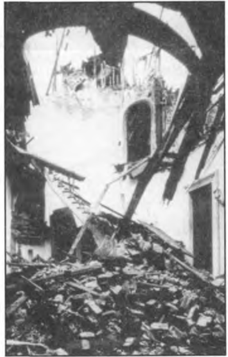
Figure 3 (left). The stair hall in a newly restored Gothic Revival board-and-batten plantation house in South Carolina, when HABS arrived to photodocument the building. Figure 4 (right). Two months later, the stair hall and 50% of the house had been reduced to rubble by fire.
